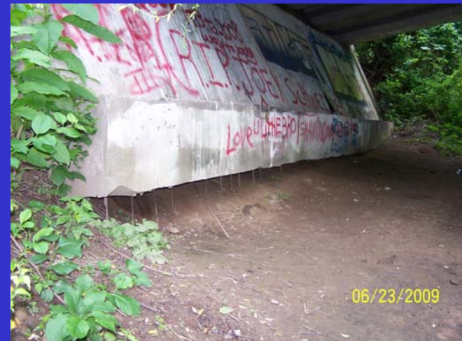
Scantic River Scour Along Bridge West Abutment
