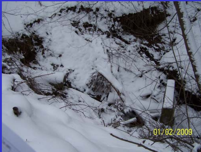
Headwall Failure (Adjacent to Holy Family Church Driveway)
