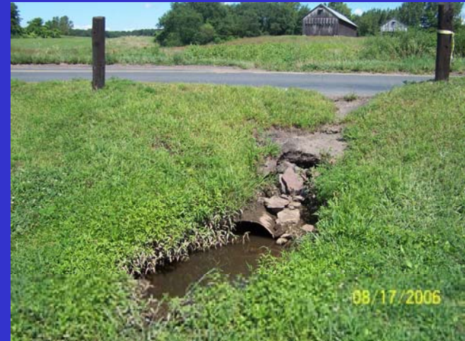
Erosion at Cross Culvert (Hazardville Water Co.)
