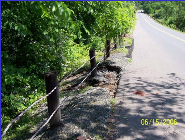
Typical Erosion Along the Roadway
